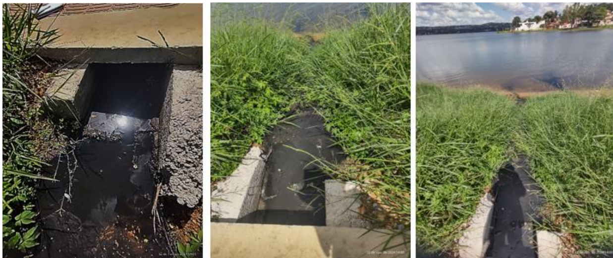
Figure 10. Effluent discharge identified at reference point P.32 (E615,085; N7,827,635; 23S).
